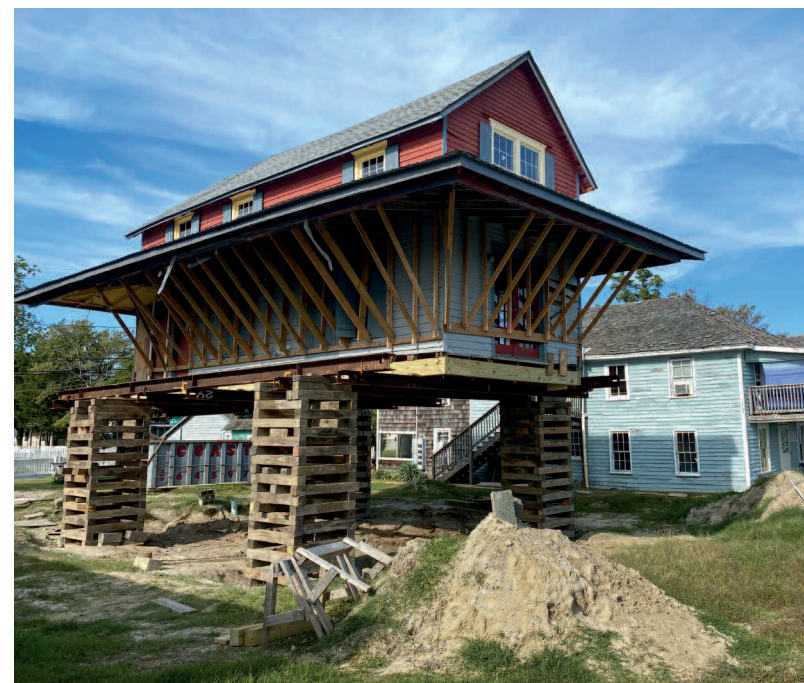
Temporary support beams bristle under the porch roof of a house being raised by Expert House Movers on River Road in Oak Orchard, which is a hot spot for flooding in Sussex County.
