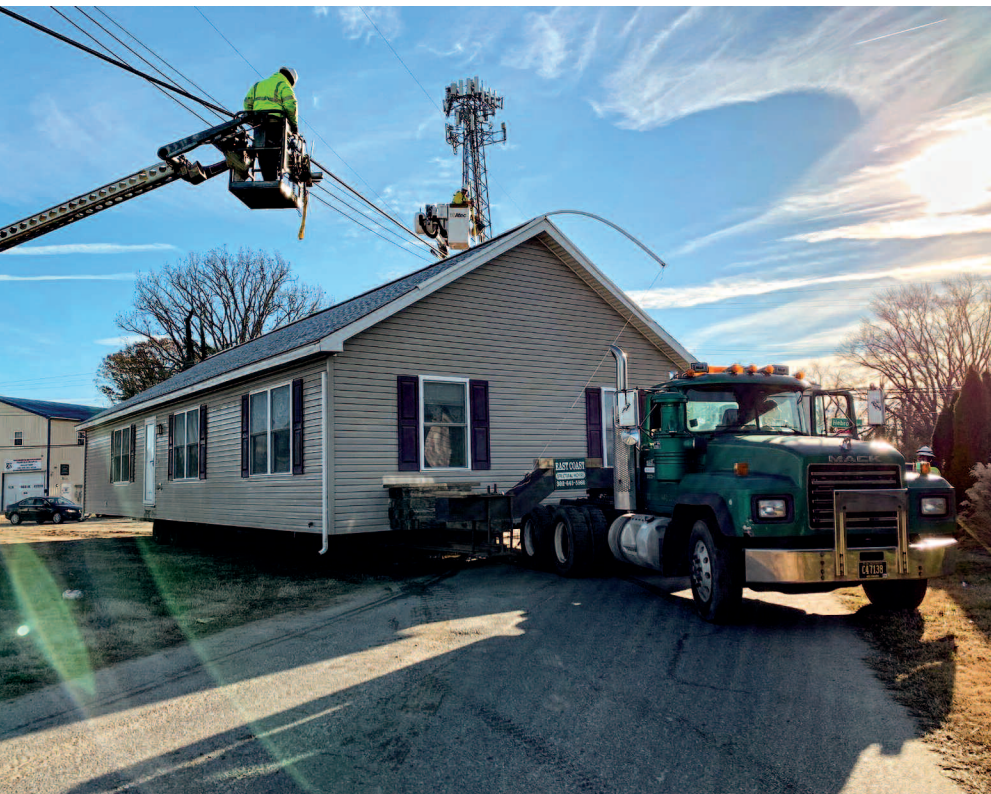
A worker lifts telephone lines, allowing this house-on-wheels to clear them during a daytime move. The curved pipe extending from the roof peak safely slides loose-hanging wires up to the roofline.
