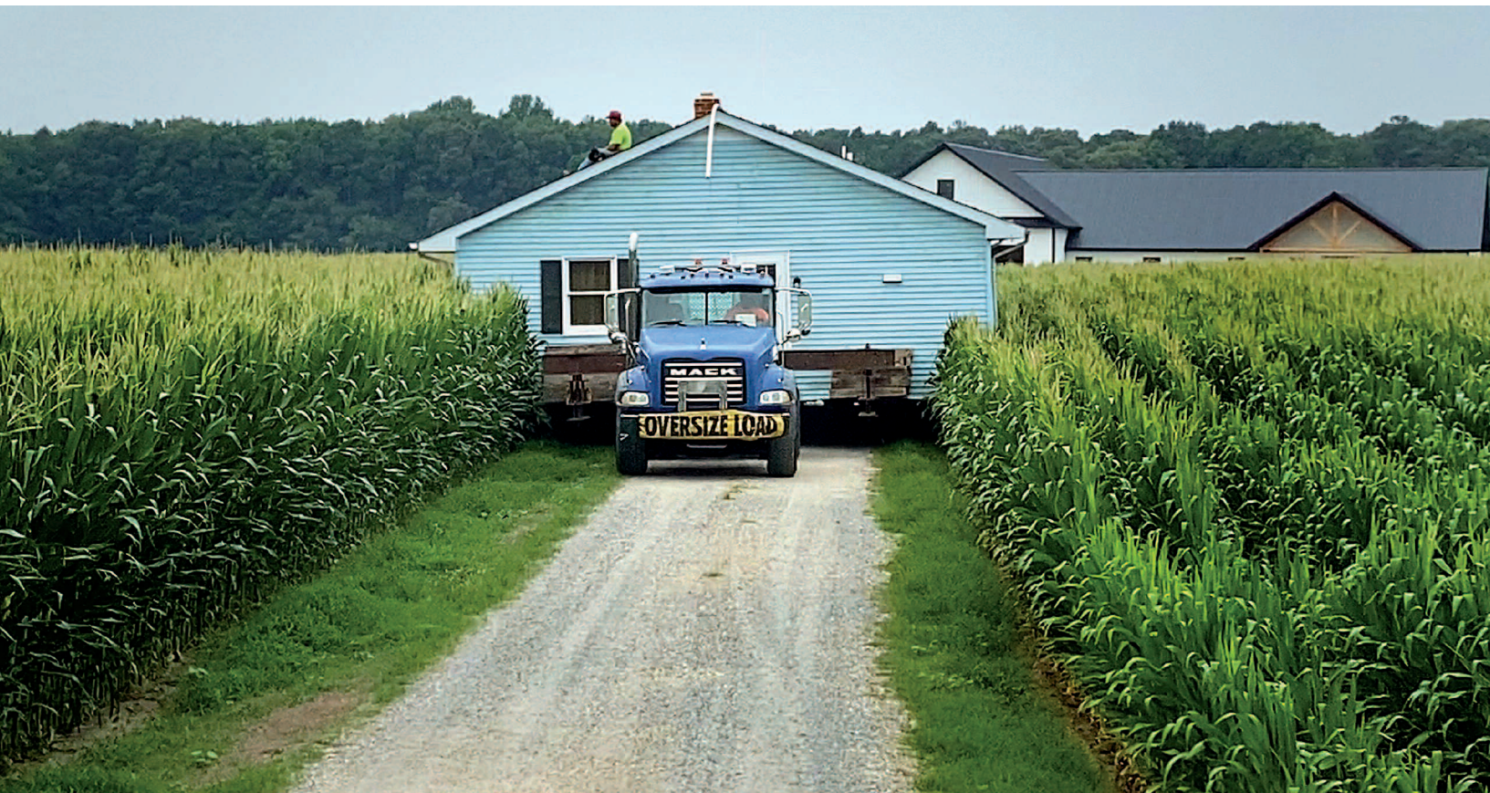
Some inconvenient rows of corn take a hit from a wide load as Expert House Movers relocates a one-story house. Rural buildings will often be moved during daylight, but in towns and along highways, the threat of traffic snarls generally makes large-scale structural projects a late-night activity.
