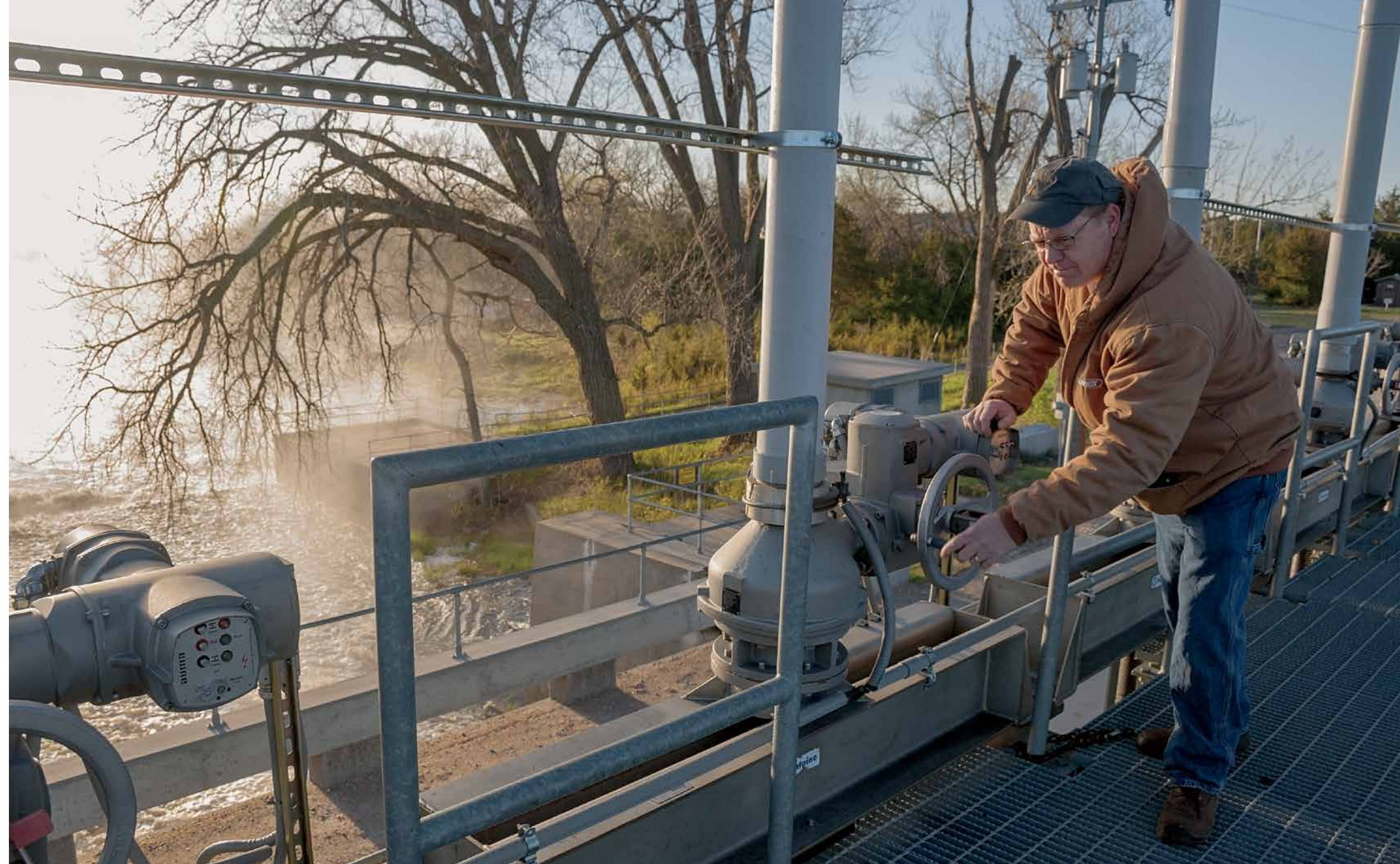
A cloud of spray erupts from the spillway below Lake Ericson as Joe Wadas of Ord makes adjustments to the dam first built a century ago.
